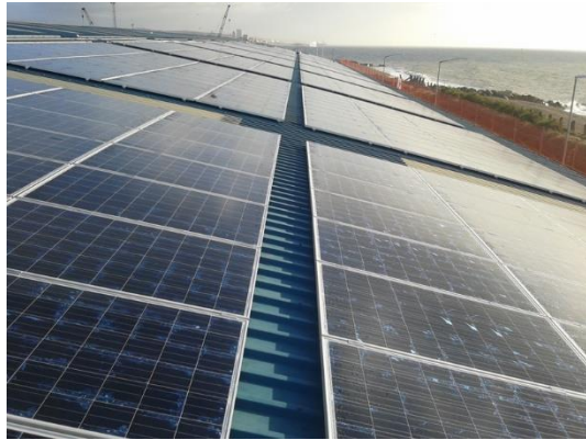
Solar panels on warehouse roofs
